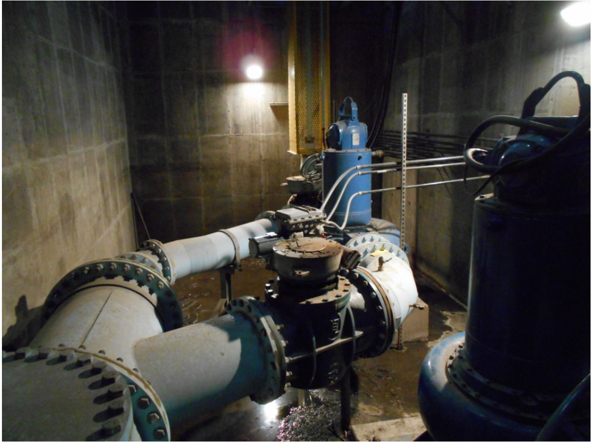
FIGURE 4-3 LIFT PUMPS NO. 2 & 3
