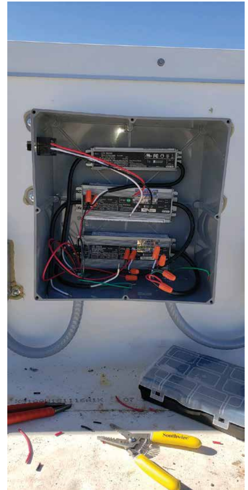
Main power box to hold LED power supplies Electrician to run main power to box for final hook up
