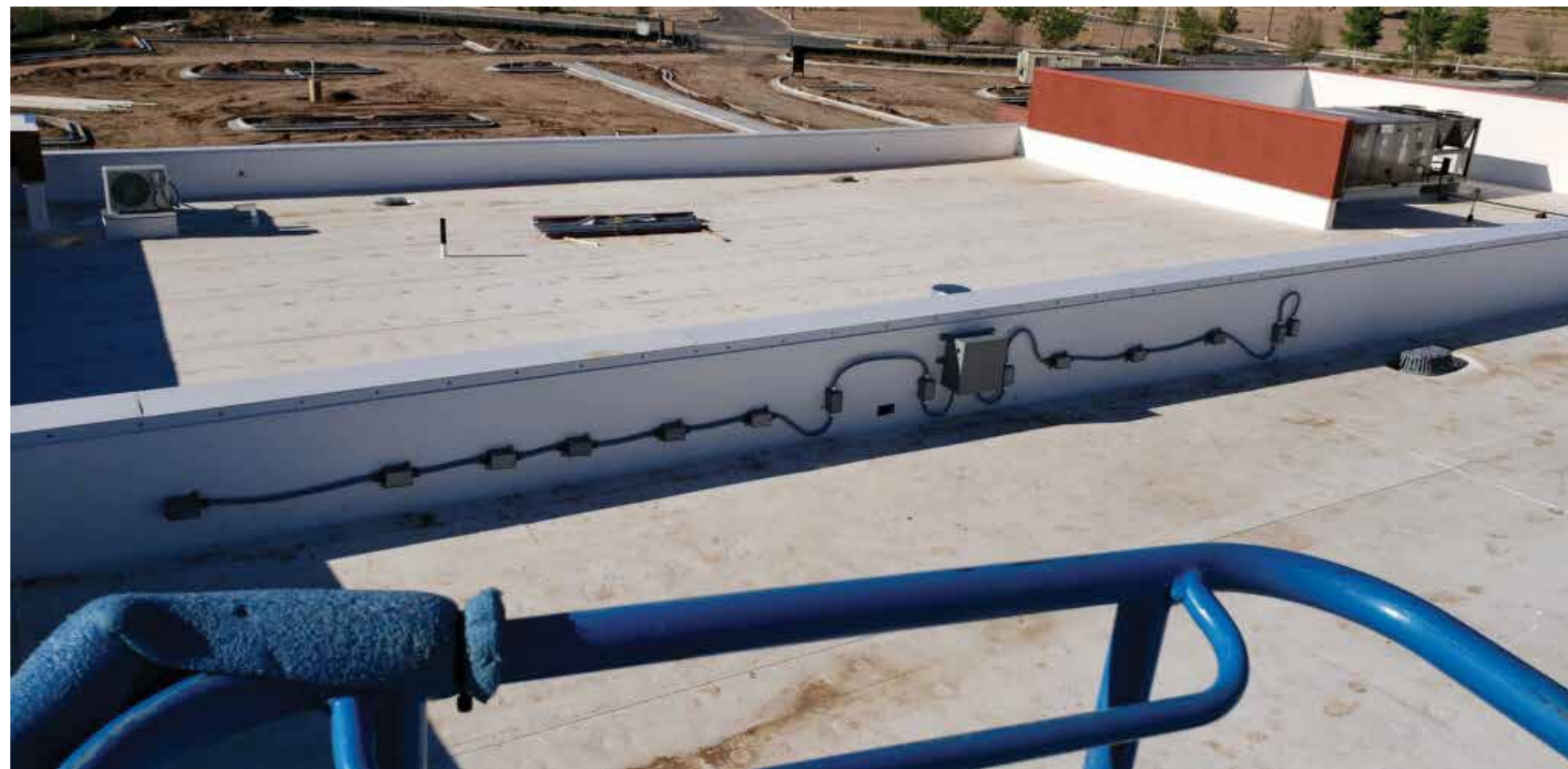
Final electrical set-up
