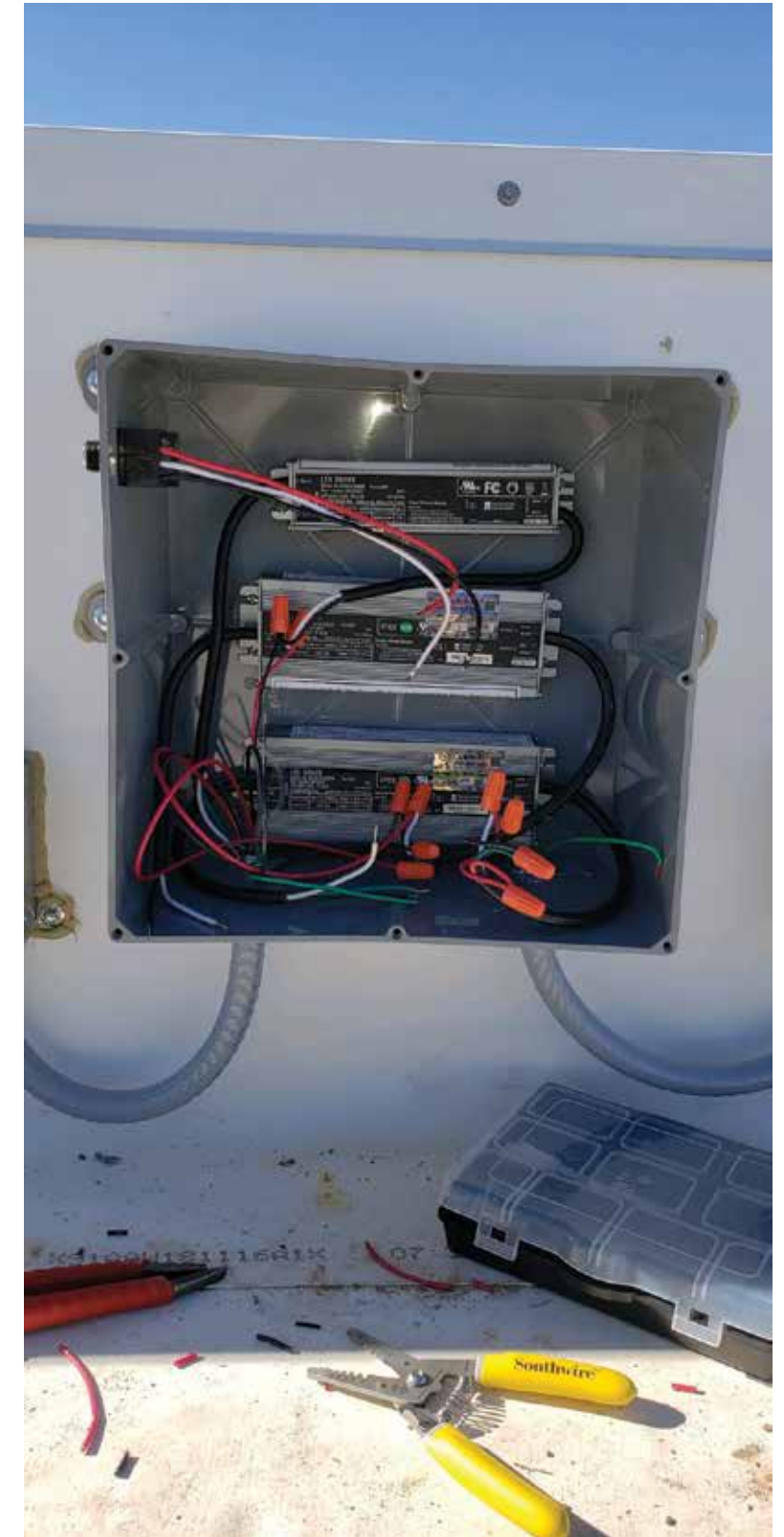
Main power box to hold LED power supplies Electrician to run main power to box for final hook up
