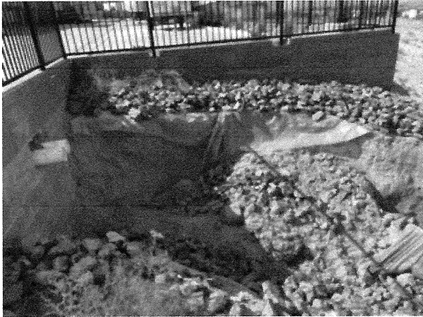
An outlet from the property to the east flows into a channel with rock lining and dirt.
