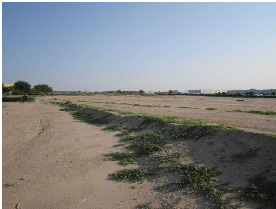
Exhibit 2: View northeast from the church parking lot of access road and depth of the excavation in the southwest corner of the survey area.
