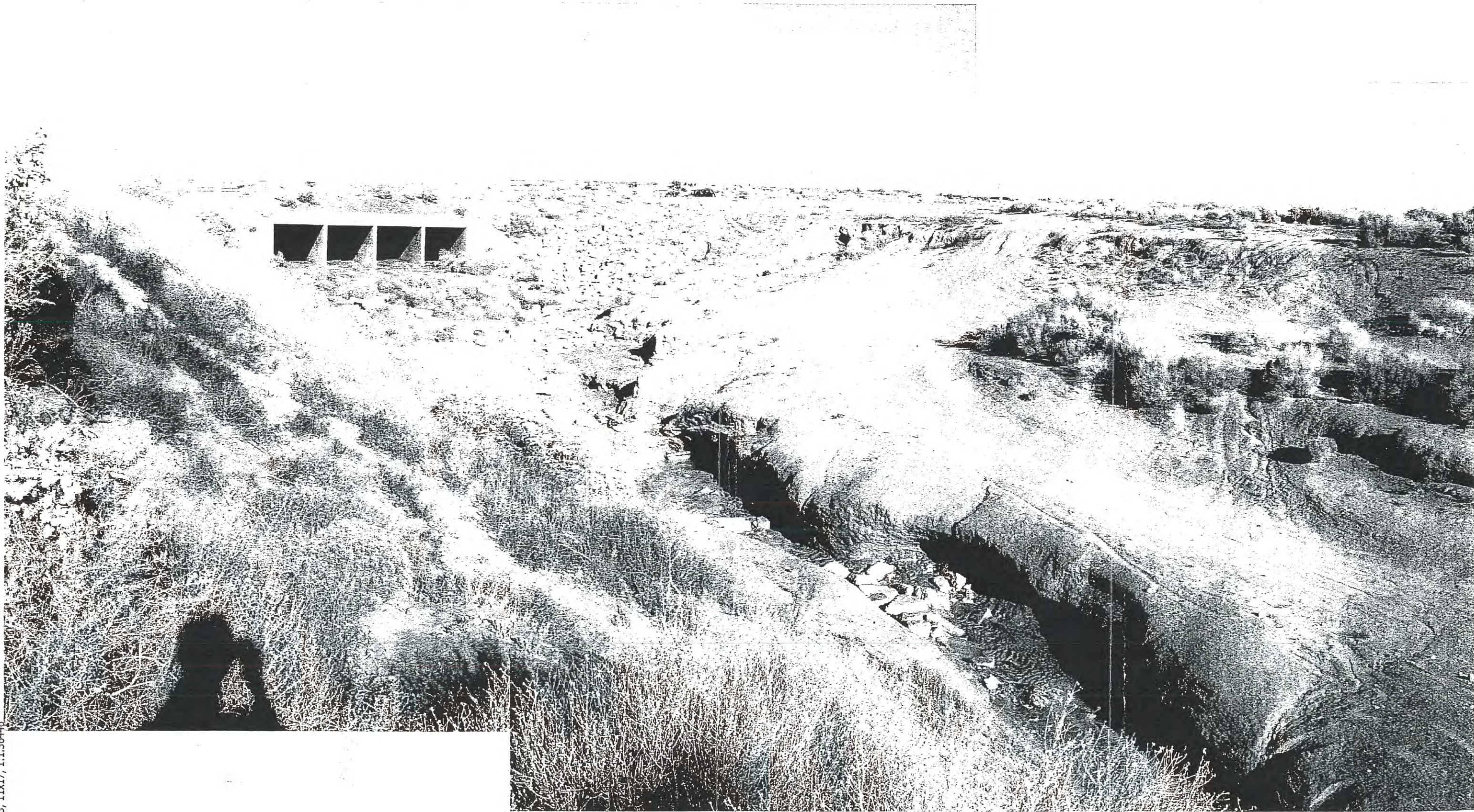
Box Culverts - Unser Blvd. Eroded Arroyo to be regraded
