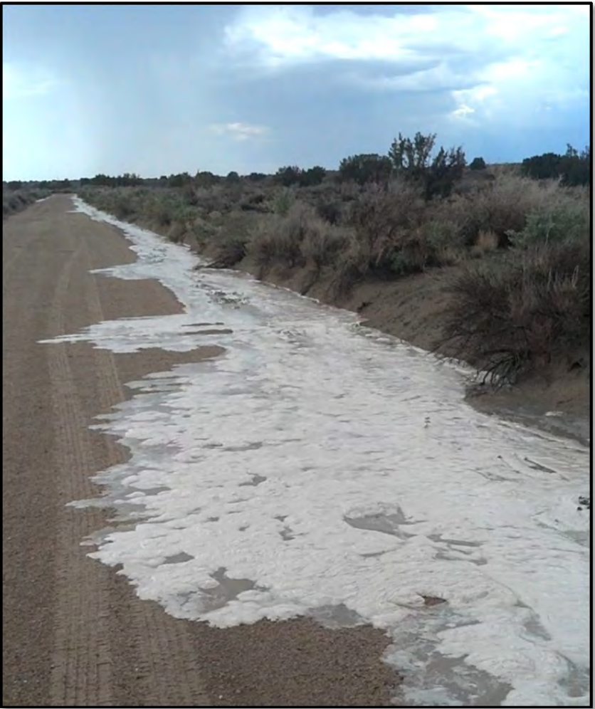
Photo 3: Picture showing a graded dirt road in the Calabacillas Watershed acting as a channel after a small storm event in August of 2013.
