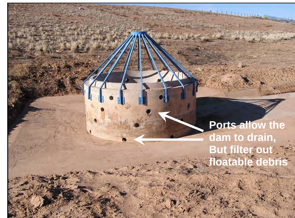
Photo 37: Water Quality outlet structure in one of SSCAFCA's flood control dams; the ports in the standpipe let water drain, but filter out floatable debris.
