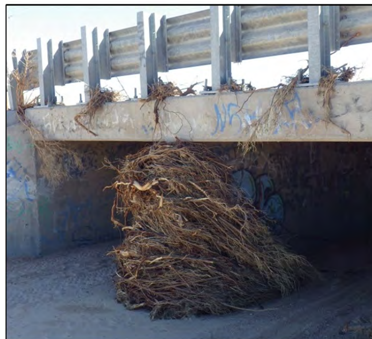
Photo 21: Debris accumulated on the upstream side of the Southern Blvd crossing following the 9/13/2013 flood.
