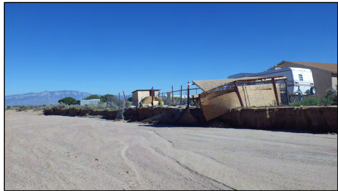
Photo 14: House built within the lateral erosion envelope of the Calabacillas Arroyo (looking east towards the Sandia Mountains in the background).
