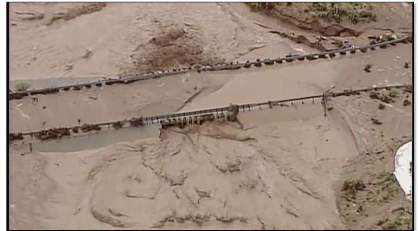
Photo 22: Storm flows overtopping Southern Blvd during the flood of September 13, 2013. (Source: KOAT News).
