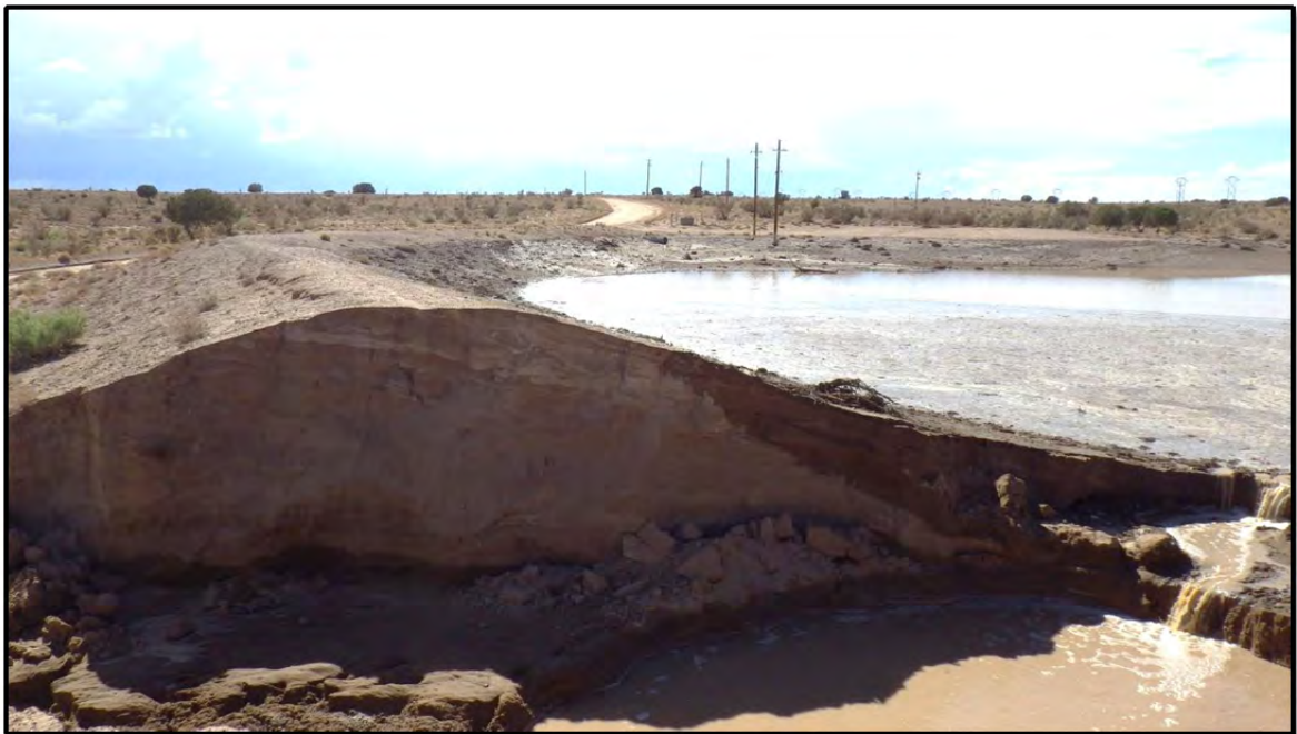
Photo 10: Stock pond north of King Blvd in Tributary N; the breach in the embankment caused by the storm of August 4, 2013 is evident in the foreground.
