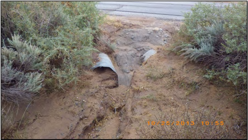
Photo 30: Culverts at Southern Blvd & Tributary C filled completely with sediment (capacity = 0 cfs).
