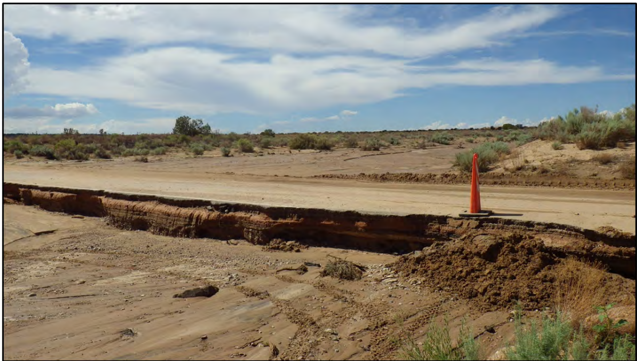
Photo 18: Damage to Northern Blvd caused by the August 4, 2013 storm.
