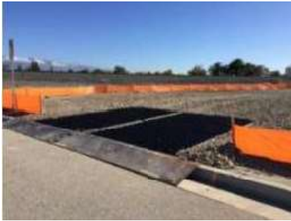
SEDIMENT TRACK OUT CONTROL
