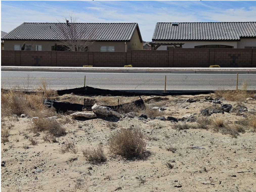
Site Walk Deficiency Photos - Inlet inside silt fence near rosa parks
