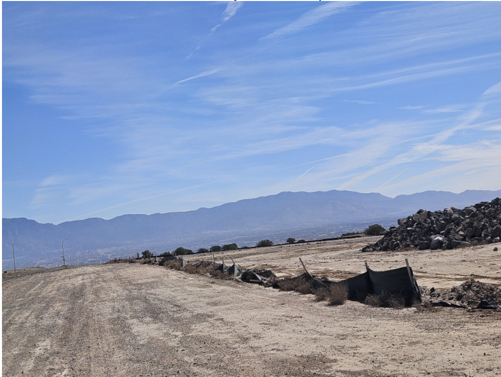
Site Walk Deficiency Photos - North perimeter
