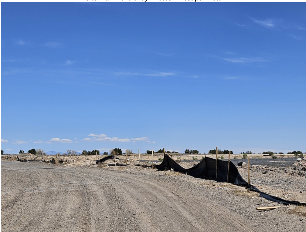
Site Walk Deficiency Photos - West perimeter
