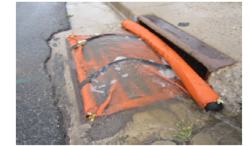
Storm drains and curb inlets should be protected with filter fabric and filter socks, which trap sediment and allow water to flow through. Photo Credit: PG Environmental for USEPA
