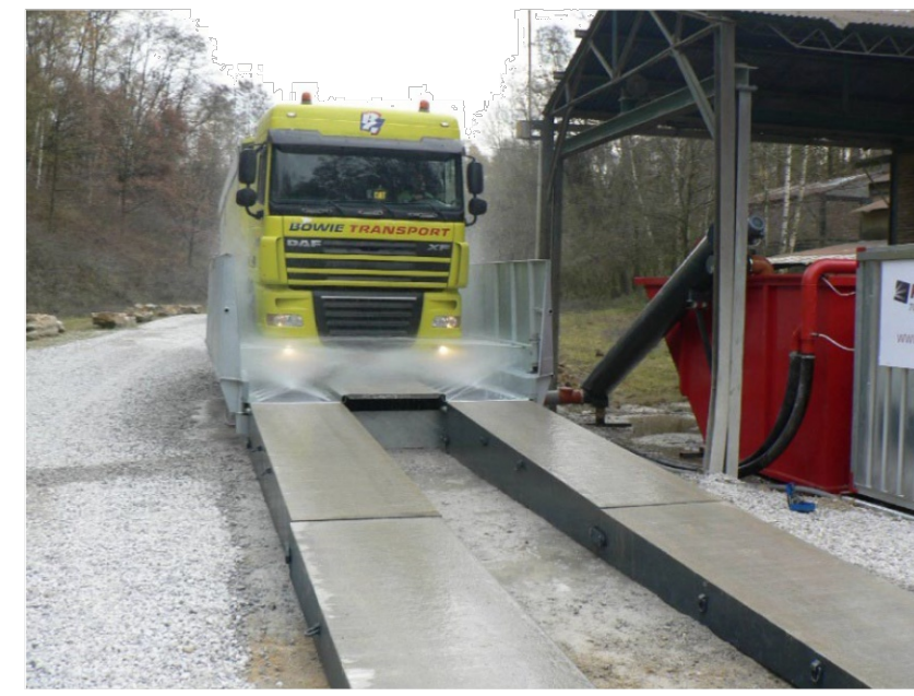
INSTALL FODS ACCORDING TO THE MANUFACTURER'S SPECIFICATIONS. FODS TRACKOUT CONTROL MATS CAN BE USED WITH A STABILIZED CE OR ALONE, AS LONG AS THEY CAN ACCOMMODATE THE TURNING MOVEMENTS OF THE LARGEST VEHICLES EXITING THE SITE.
