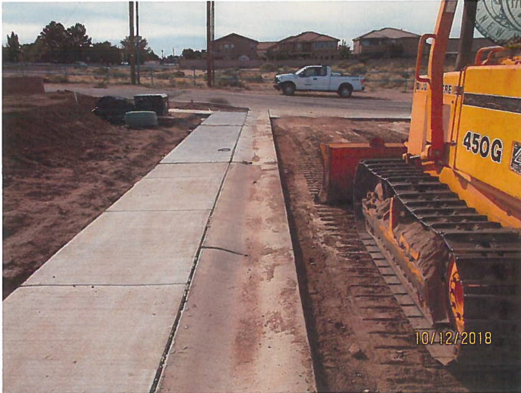
East gutter- No sediment BMP
