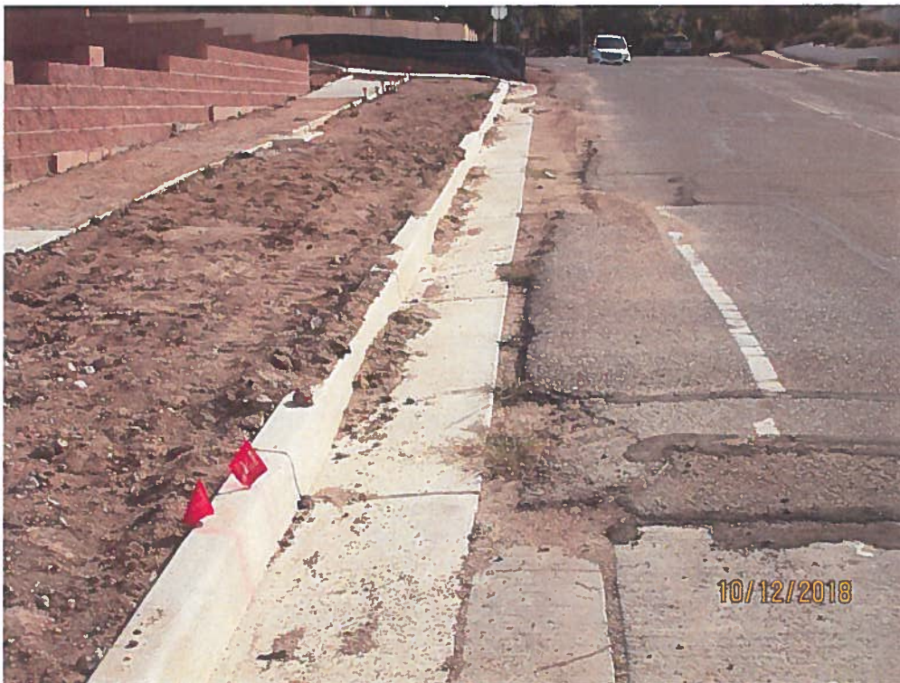
Sediment in gutter and on top of curb.
