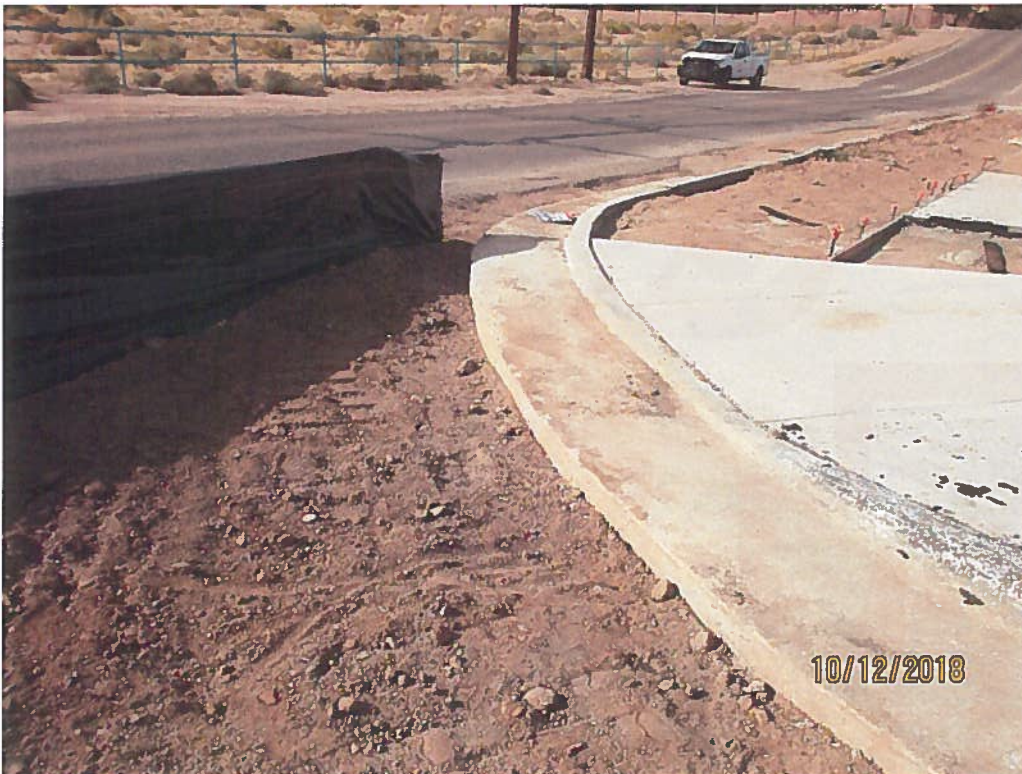
Wyoming south end- No sediment BMP for gutter and gap next to gutter.
