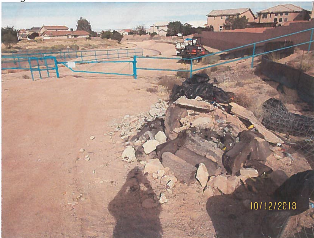
Construction waste and litter pile near channel.
