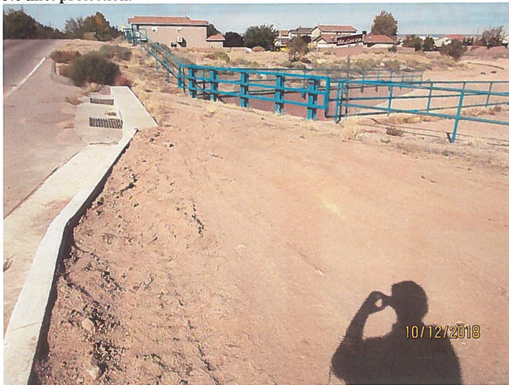
Disturbed area uphill from channel with no sediment BMP.
