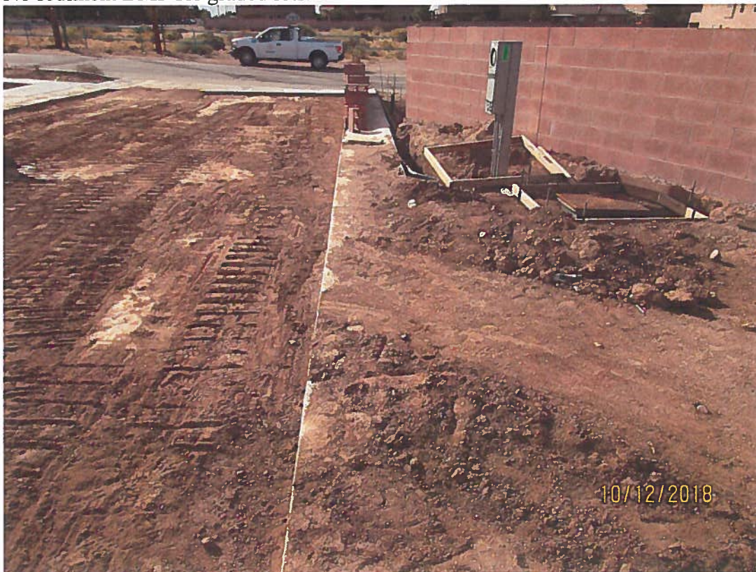
West gutter-No sediment BMP.
