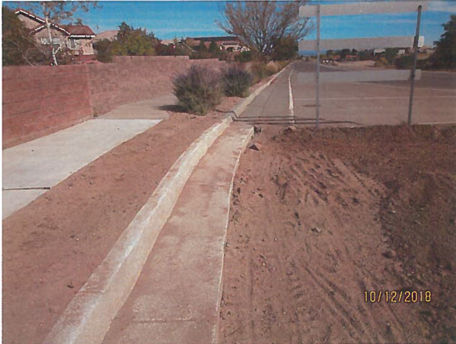
Wyoming Blvd North end-no sediment BMP.
