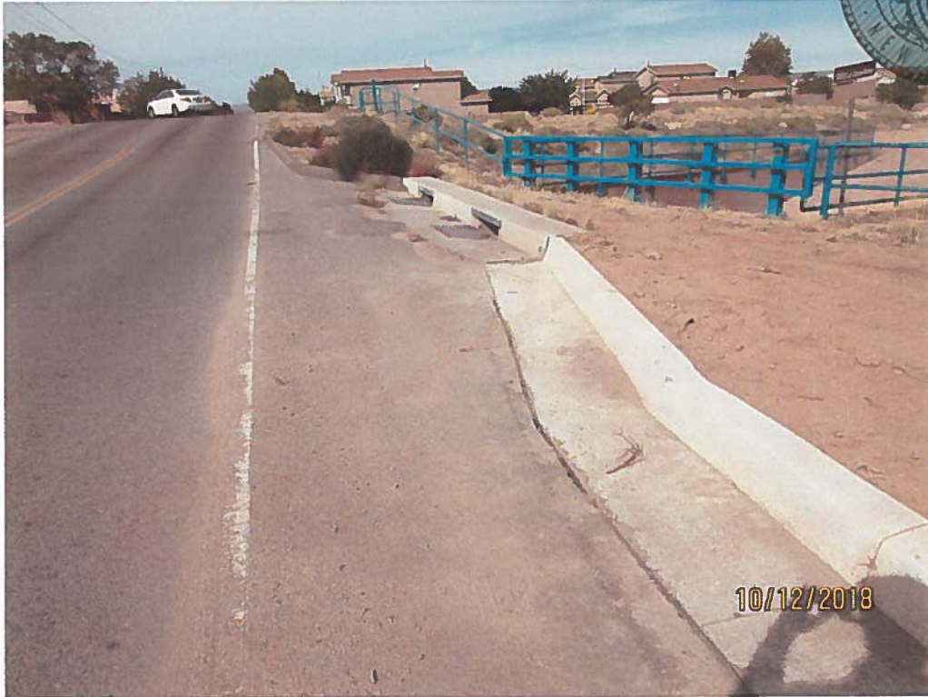
No inlet protection.
