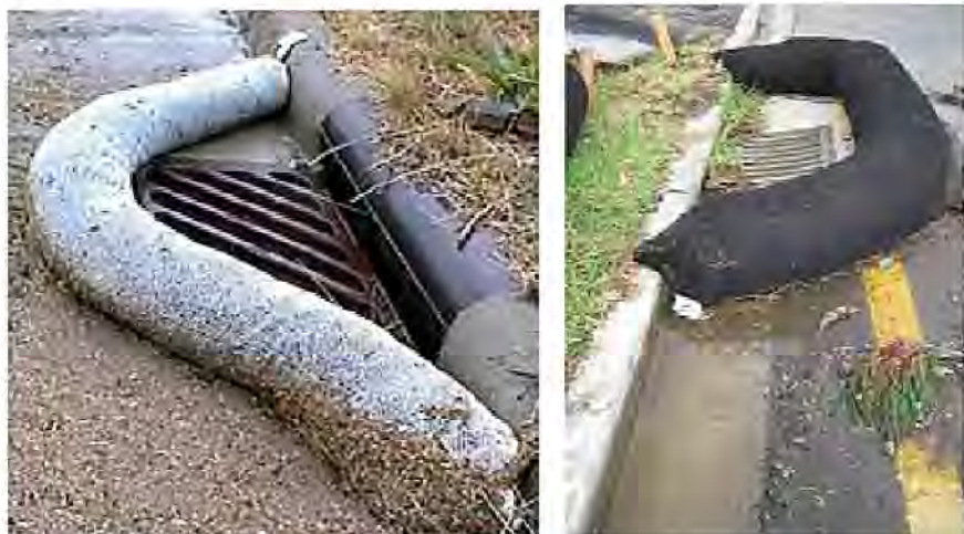
Curb Storm Inlet Protection with Wattles
