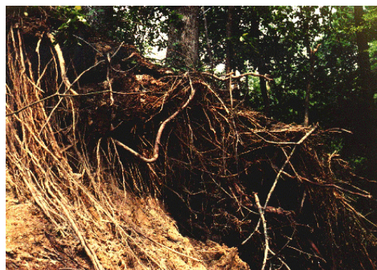
Figure 8. Exposed tree roots in overtopped dam.
