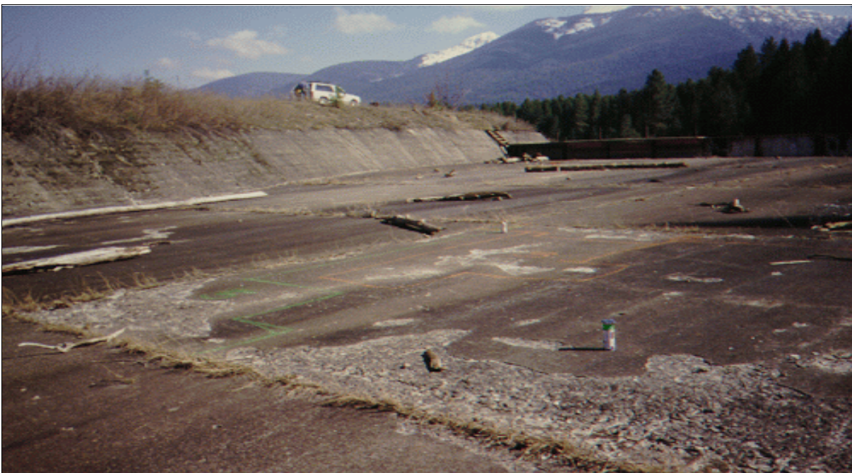
Figure 21.—Freezing and thawing deterioration on spillway concrete.
