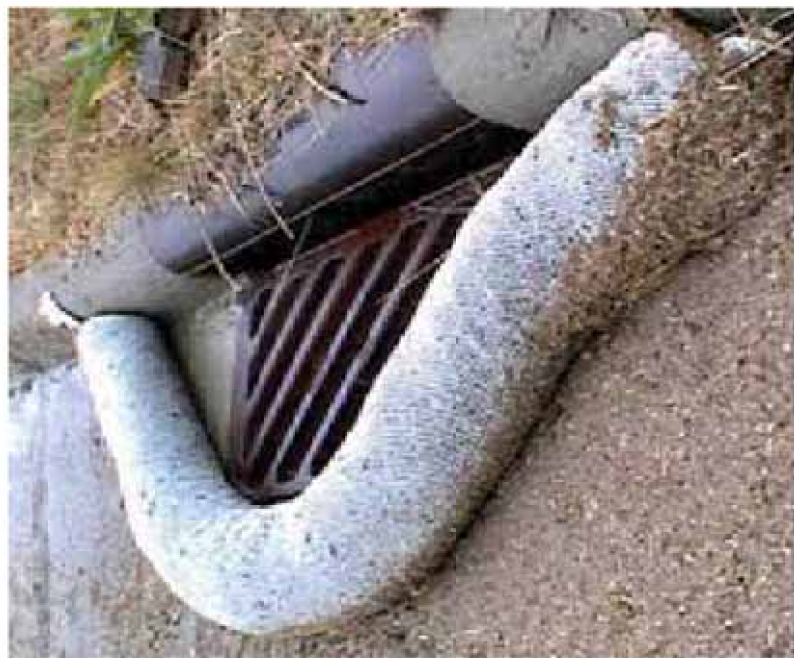
Curb Storm Inlet Protection with Wattles
