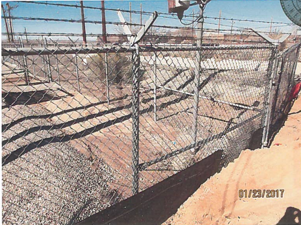
Gap in silt fence and sediment on adjacent property.
