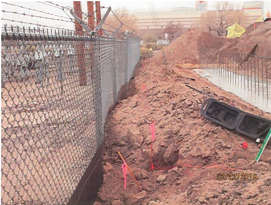
Dirt piled-up against silt fence.
