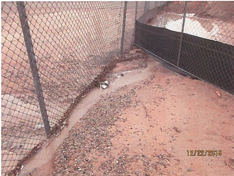
Drainage leaving site.
