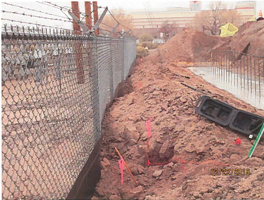
Dirt piled-up against silt fence.
