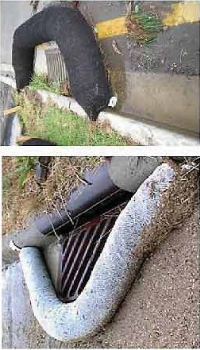
Curb Storm Inlet Protection with Wattles
