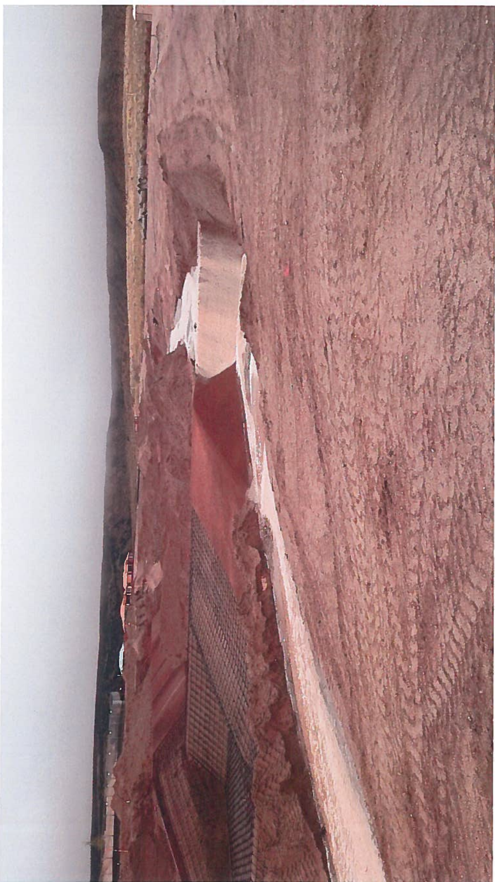
Piles of loose dirt eroding.
