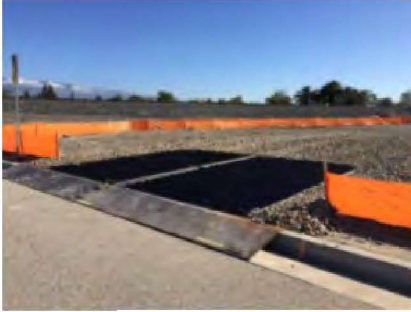
SEDIMENT TRACK OUT CONTROL
