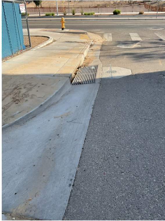
Site Walk Deficiency Photos - North east corner
