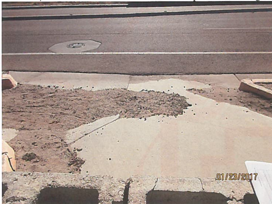
Sediment on ADA ramp/sidewalk.
