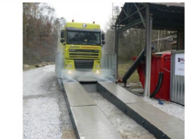
INSTALL FODS ACCORDING TO THE MANUFACTURER'S SPECIFICATIONS. FODS TRACK-OUT CONTROL MATS CAN BE USED WITH A STABILIZED CE OR ALONE, AS LONG AS THEY CAN ACCOMMODATE THE TURNING MOVEMENTS OF THE LARGEST VEHICLES EXITING THE SITE.
