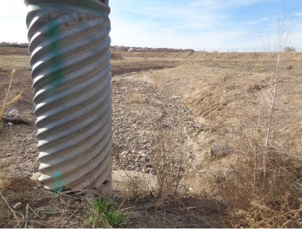
Figure 7 - Erosion from Modified Outfall
