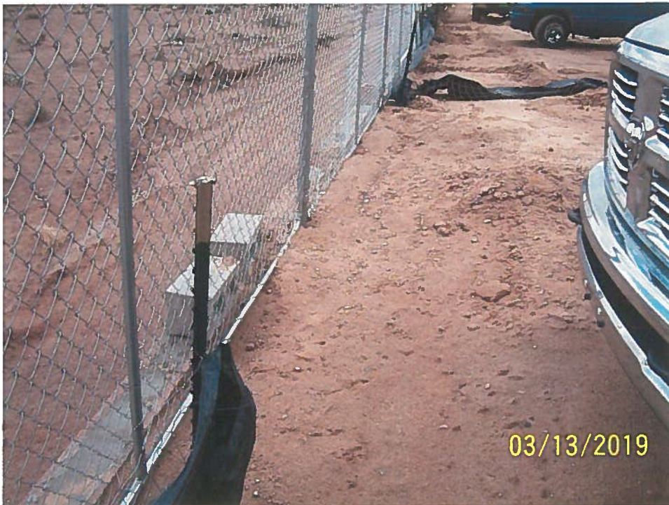
Gap in silt fence.
