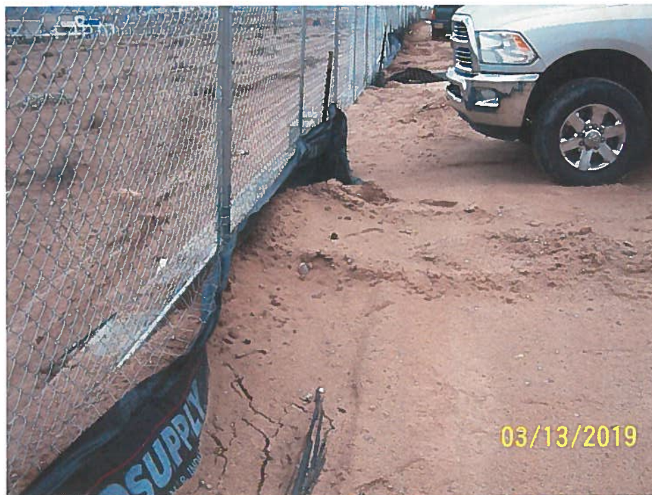
Silt fence not buried.
