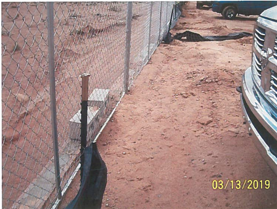
Gap in silt fence.
