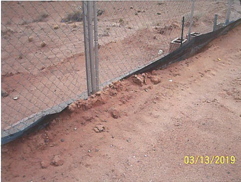
Grade higher than halfway up silt fence.
