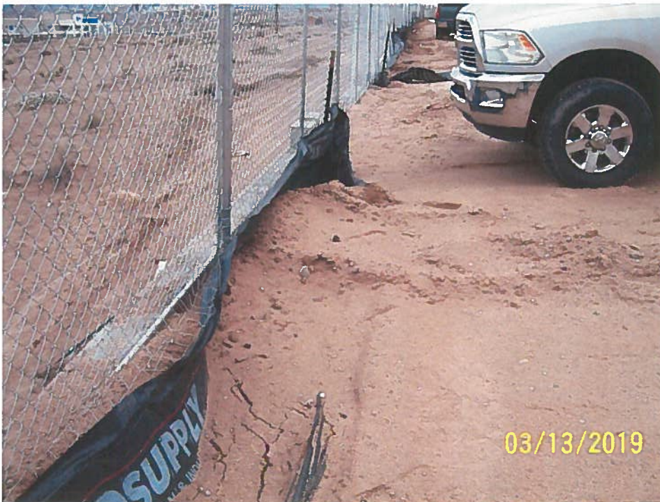
Silt fence not buried.
