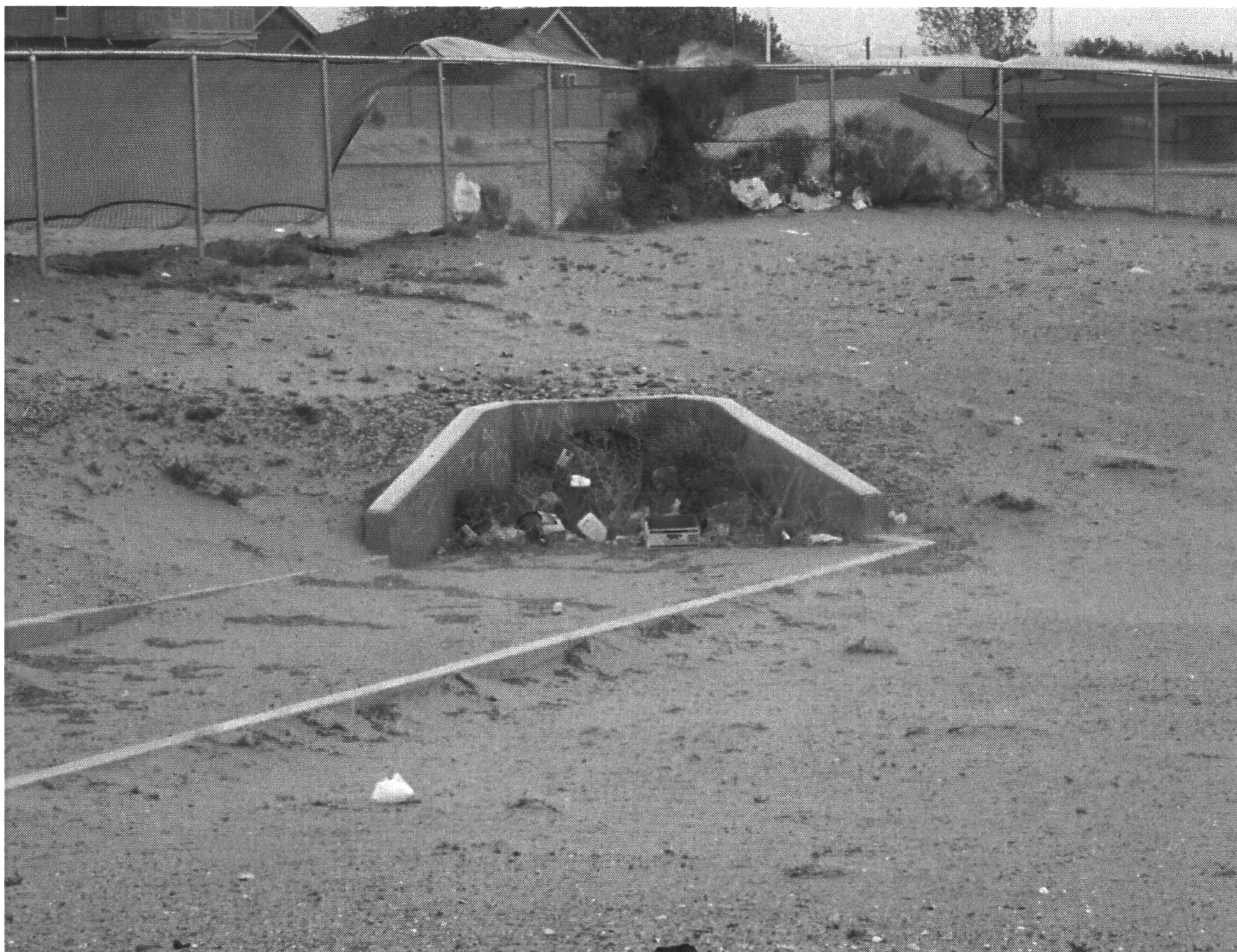
FIGURE 8: Outfall located at the northeast corner of the site. This headwall and associated culvert outlets to the Amole Channel. Routine maintenance is required to remove sediment, trash and debris.
